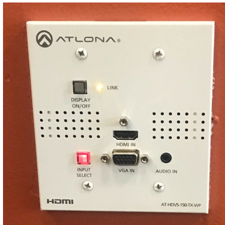
New A/V connector in West Meeting Room installed by Tel Systems
