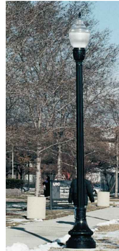
4G decorative light and pole (1-CONDITIONS)
