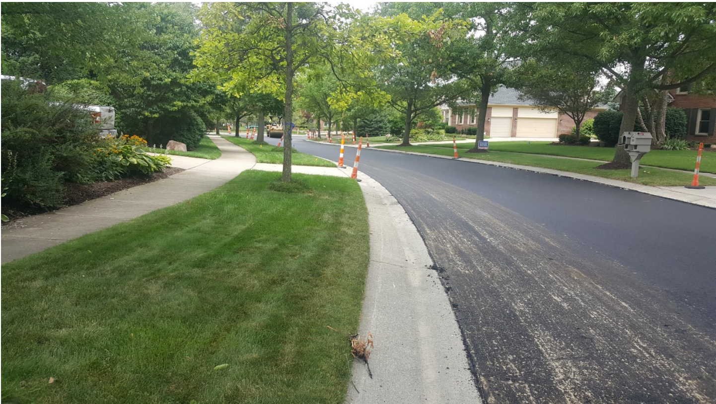
Greenwood Oaks Sub – Shilo Drive – Completion of the first lift of asphalt
