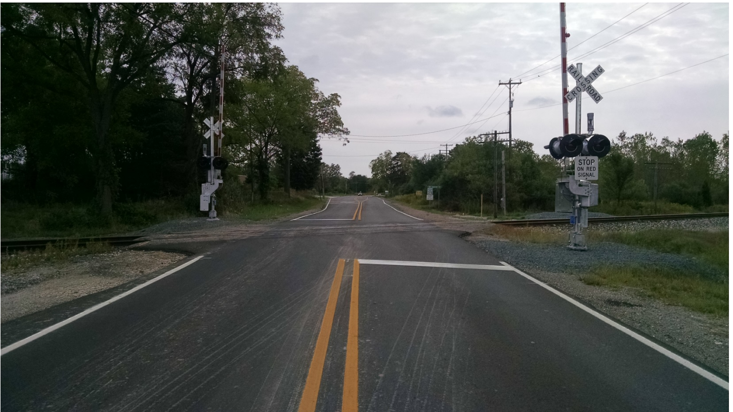
West Road – Looking east from City Limits (CSX Railroad). Full Asphalt Rehabilitation.
