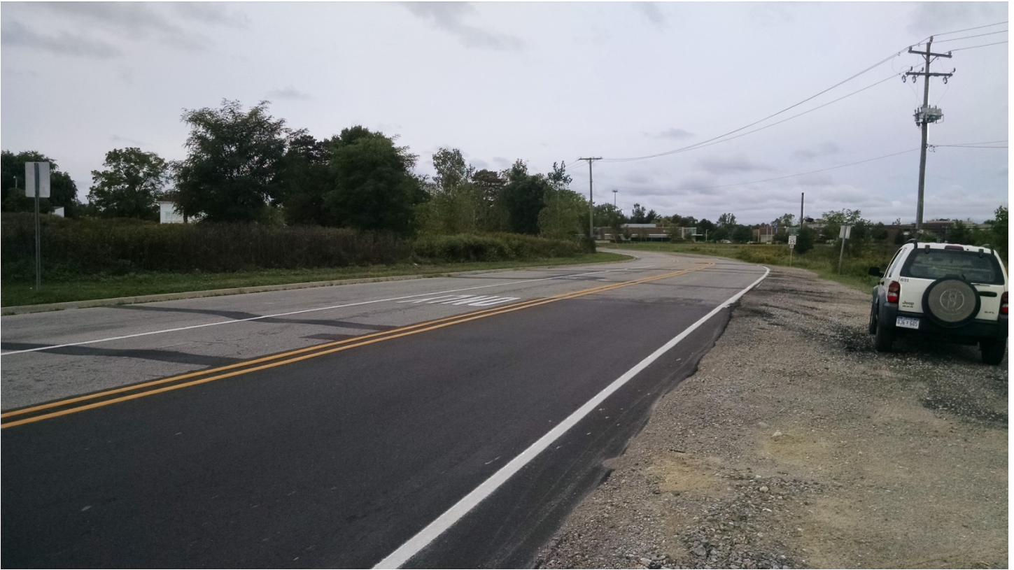
West Road – Looking west from West Park Drive. Joint Repairs and long patches.
