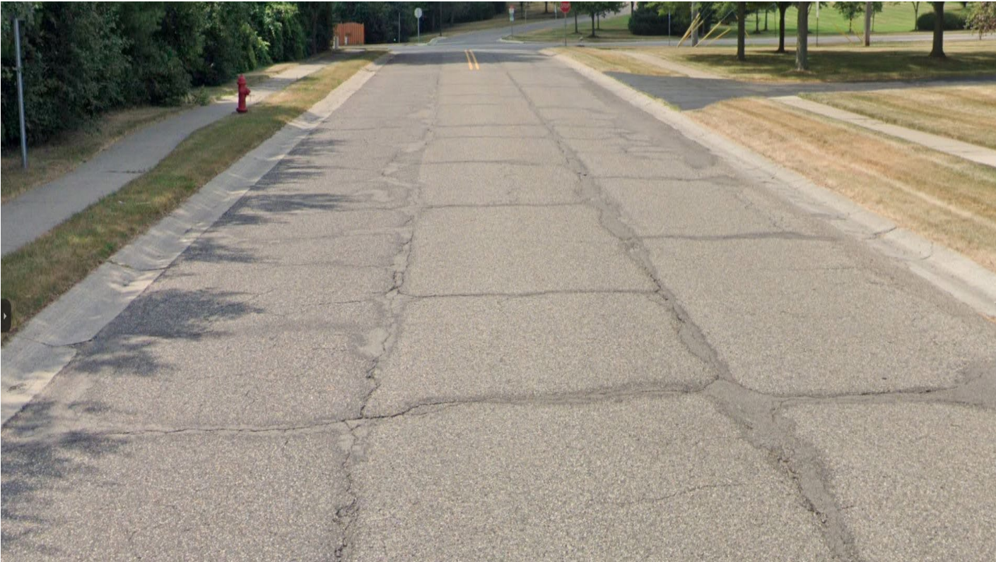
Before – Christina Lane, north of Ten Mile Road, looking south
