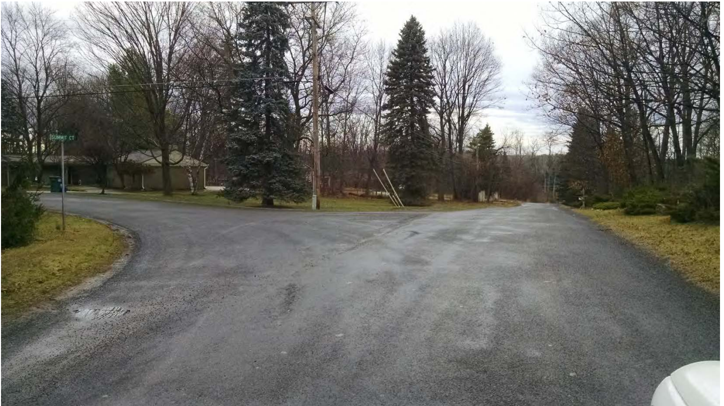
2014 Chip Seal Program – Looking North Along Summit Drive and the Intersection of Summit Court.
