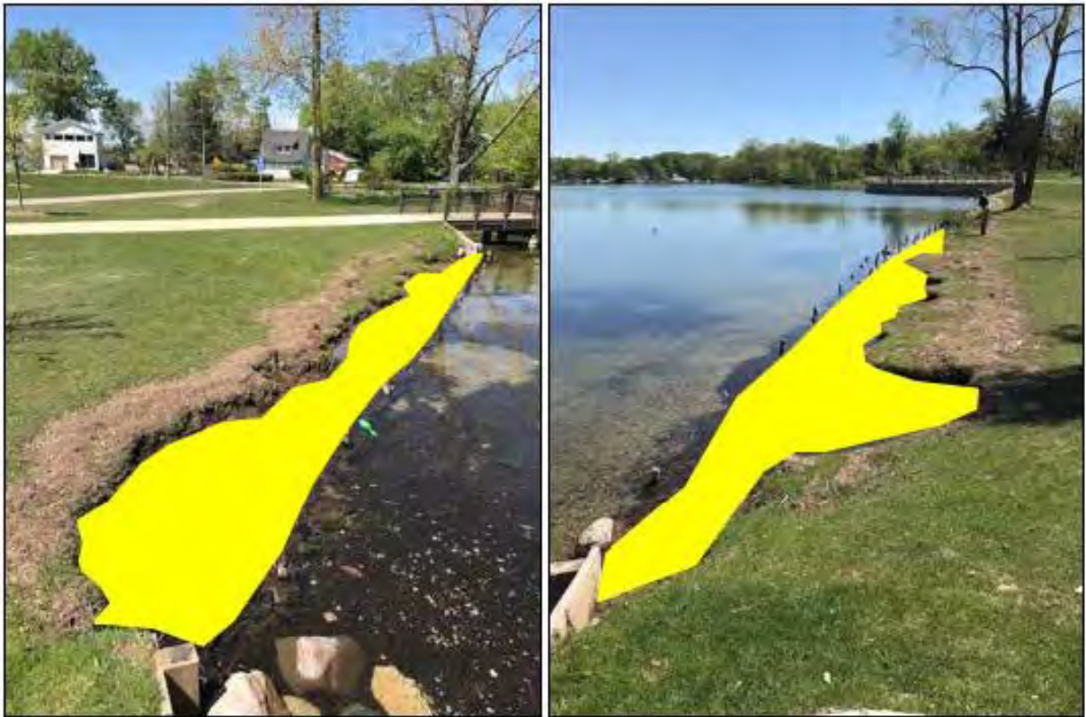
Yellow denoting the amount of area eroded |
