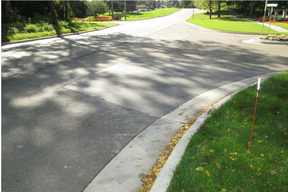
Patch and surface condition at kink in neighborhood entrance
