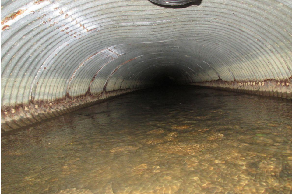
South pipe out of round
