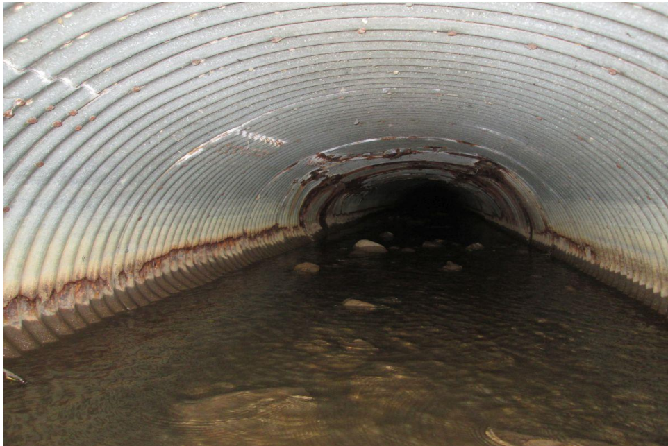
North pipe damage
