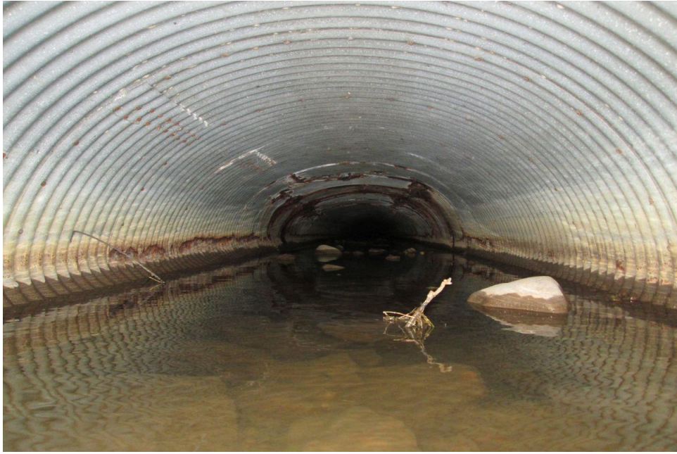
North pipe damage
