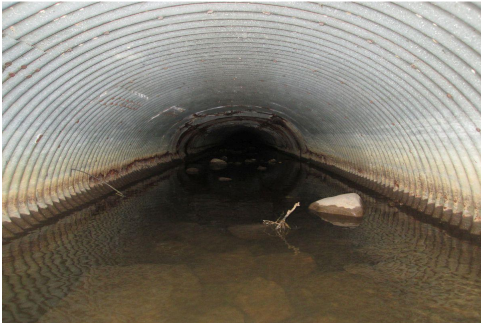
North pipe damage
