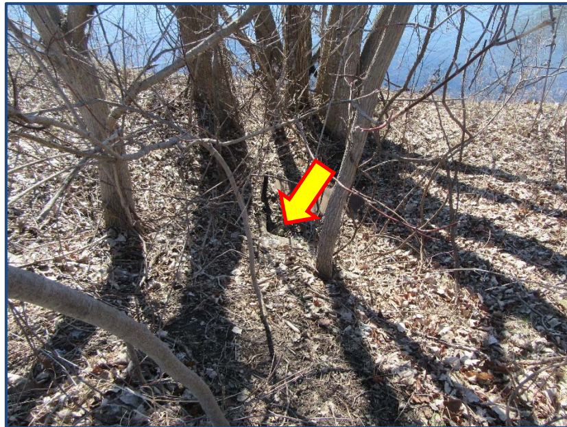
Photo 2. Existing 18" storm sewer end section located at northwest side of the pond/wetland (ECT, March 22, 2017).
