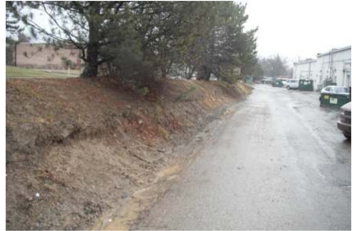
2. Rear of commercial center – Berm erosion; exposed meters, pipes, and Conduit; and unenclosed dumpsters
