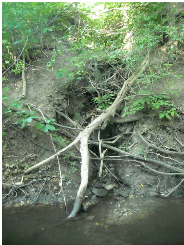
Gully Erosion along Site 7
