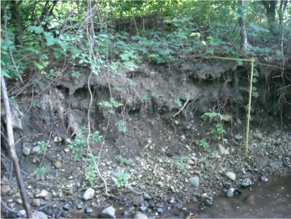
Bank Failure, Bank Height = ~ 3.5', BEHI = 34/Very High
