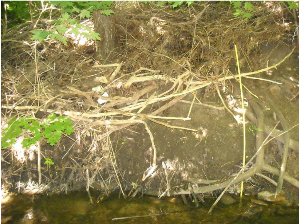
Toe Erosion, downstream end of Site 4
