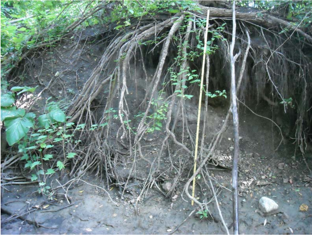
Undercutting Bank, Bank Height = ~ 7', BEHI = 29/Very High
