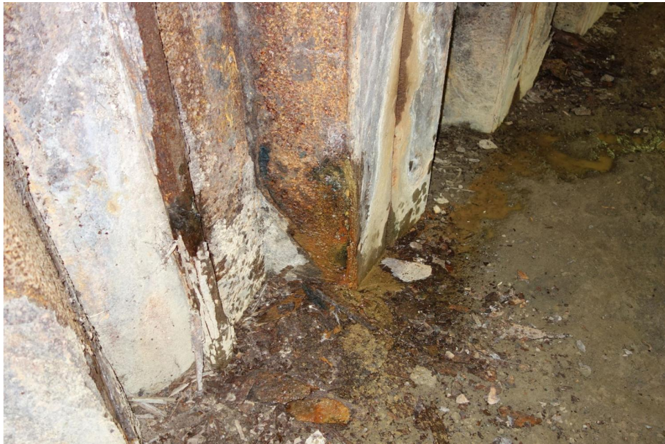
South Abutment Sheeting Section Loss and Rusting
