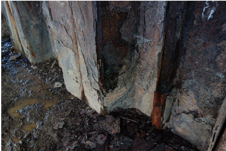
North Abutment Sheeting Section Loss and Rusting
